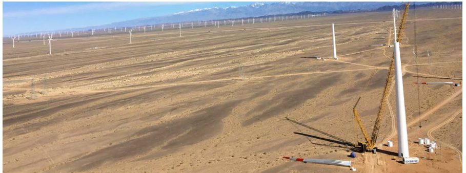
Hami Wind Power Plant
