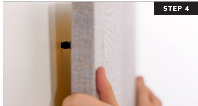
Push the panel onto the black ratchets to make indentations in the panel core material.
