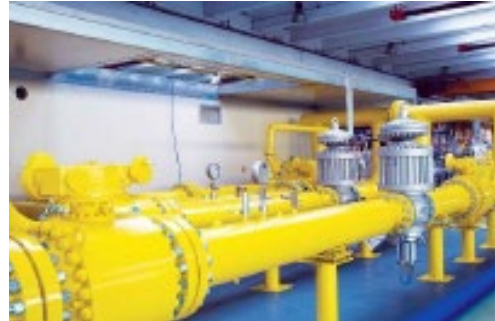
Gas Conditioning, Regulating & Metering System
