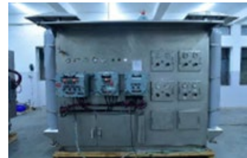
Wellhead Control Panel
