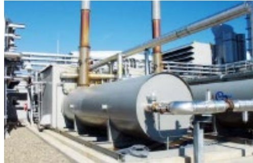
Indirect Water Bath Heater
