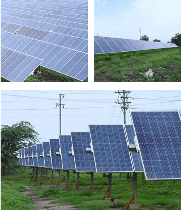
Akot, Maharashtra 14 MWp, Solar Farm
