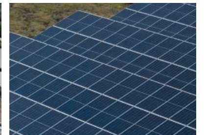
Ground Mount Solar
