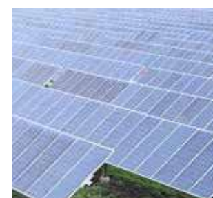
Akot, Maharashtra 14 MWp, Solar Farm
