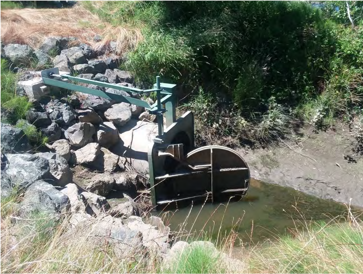
Figure 2. A 6' diameter aluminum side-binged MTR tide gate was installed at the Cochran project in 2017. The tide gate door is installed on the riverside of the culvert.
