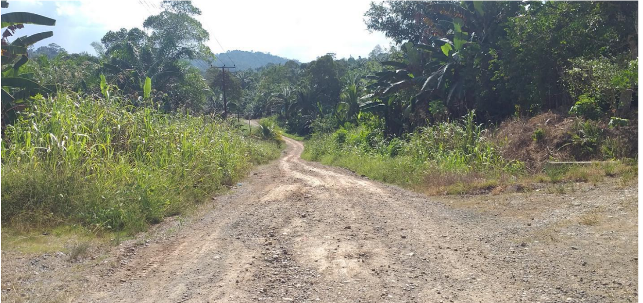
Figure 11 Gravel and unpaved road in one of the villages
