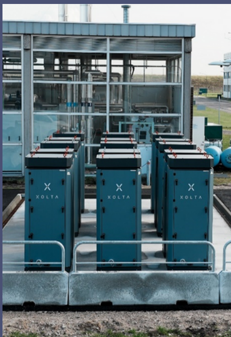
Figure 8 – Individual battery racks spaced with 50 cm.
