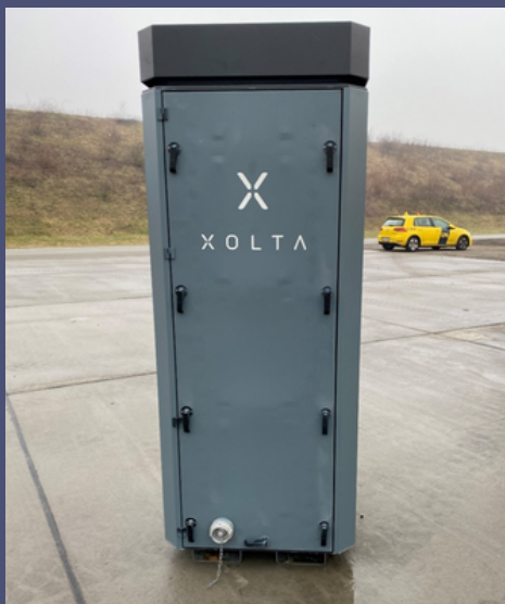
Figure 6 – Individual battery rack from Xolta. All racks are equipped with a connector for a fire hose, so they can be filled with water in case of fire.
