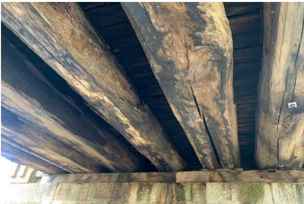
Figure 4.9: Bushfire damage to timber bridge
