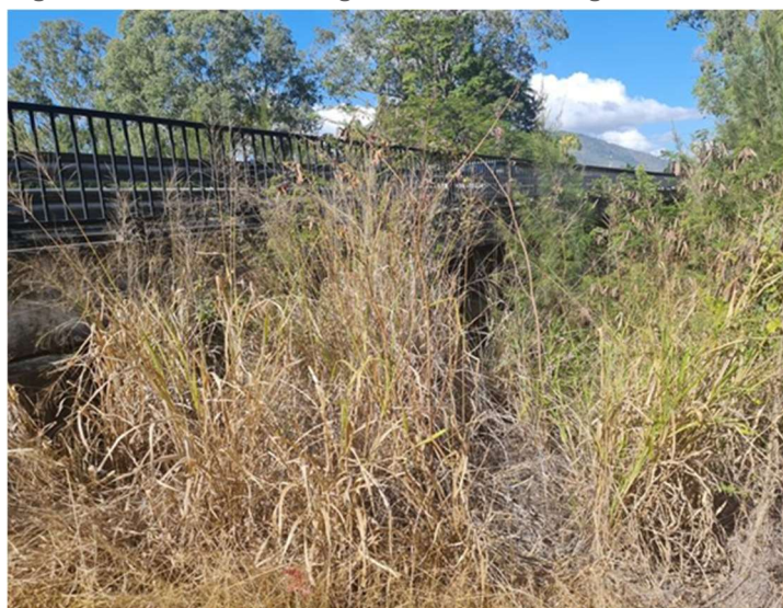
Figure 4.14: Excessive vegetation encroaching structure
