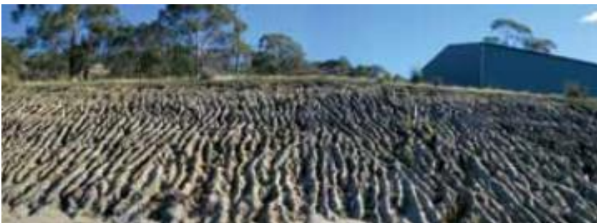
Figure 2.14: Example of rill erosion
