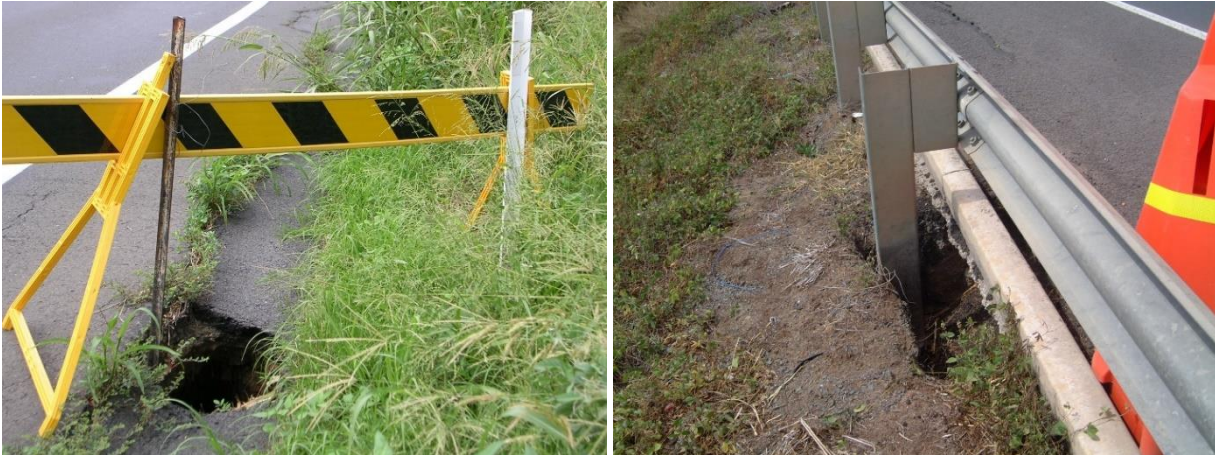
Figure 2.12: Tunnel erosion along the verge of road pavements on the Cunningham Highway
