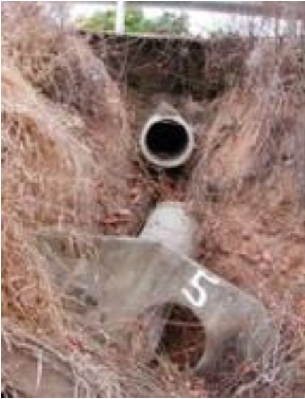
Figure 2.17: Damaged drainage structure from dispersive soils
