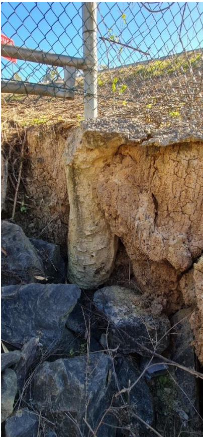
Figure 2.16: Undermining of fence footings by erosion of dispersive material
