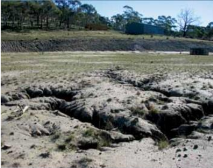
Figure 2.15: Example of tunnel erosion in footings
