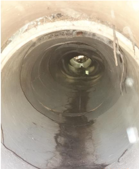
Figure 2.18: Collapsed pipe culvert on the Mt Lindsay Highway (Queensland) caused by tunnel erosion around the outside of the culvert
