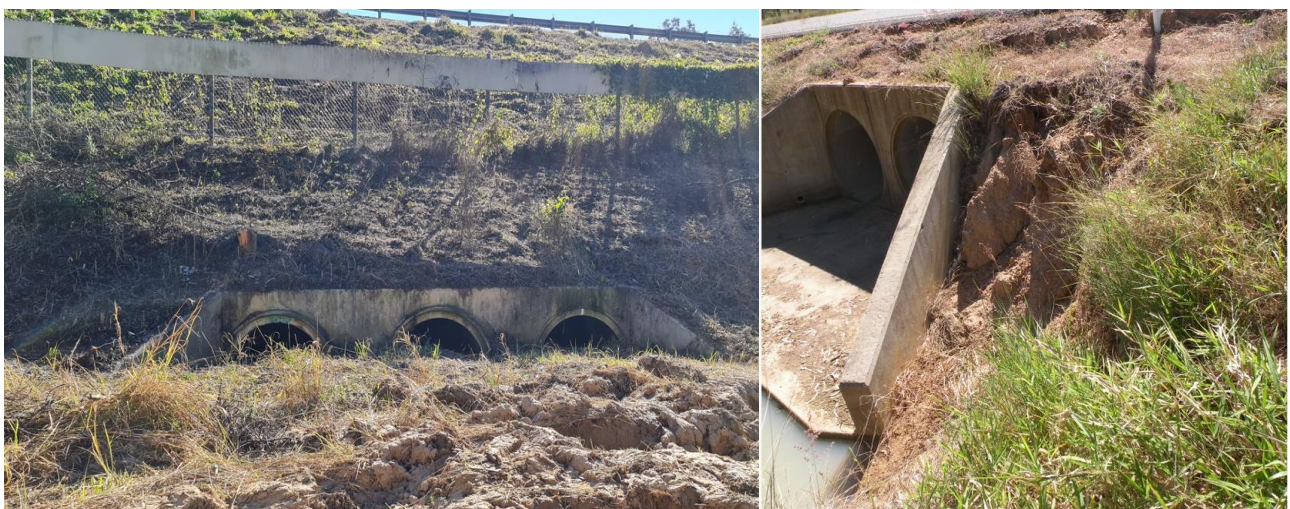
Figure 2.10: Example specification of erosion of dispersive materials and resultant deposition of sediment in culverts
