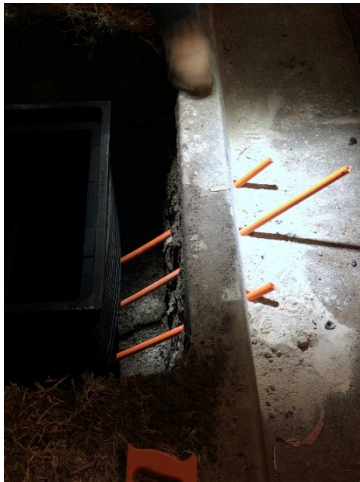
PVC conduit from the kerb into the cable pit
