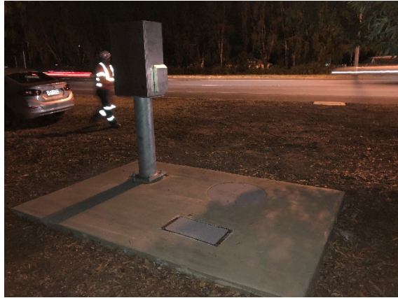
Telecommunication field cabinet
