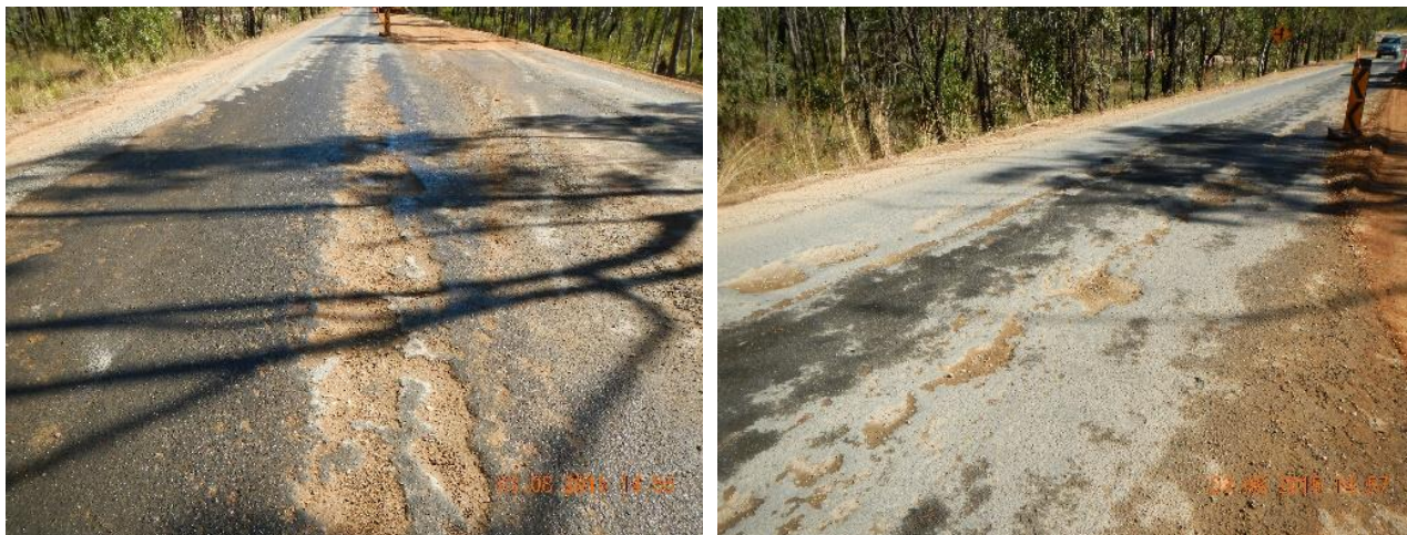
Figure 1.1: Suspected moisture-related failures of a cement modified basecourse on the outskirts of Ravenshoe, Far North Queensland
