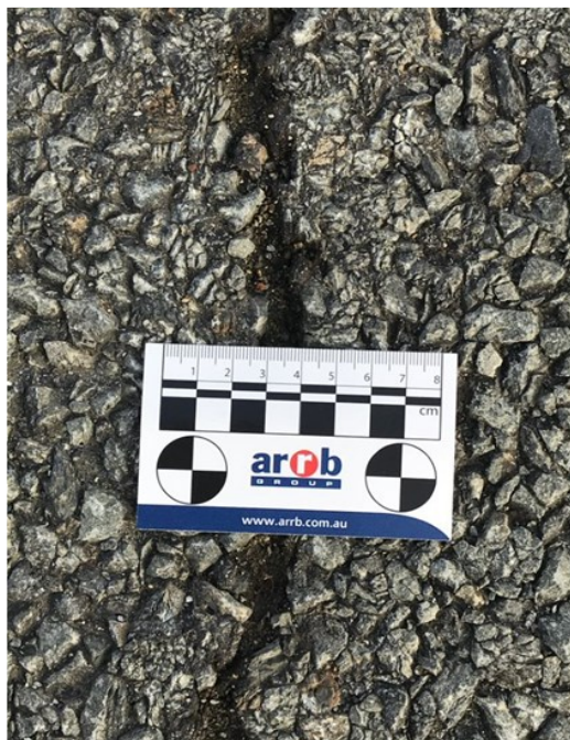
Figure 4.3: Large stabilisation crack
