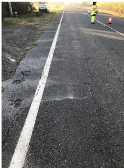
Figure 4.4: Block cracking with pumping of the fines
