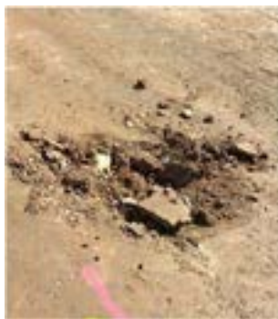
Excavations not vertically sided
