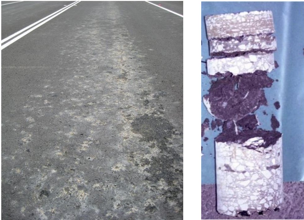
Figure 2.1: Asphalt stripping failures
