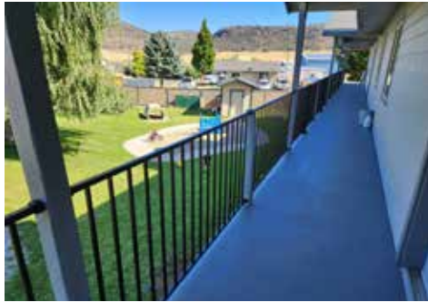
Yreka Upstairs Railing
