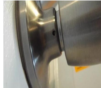
Figure 5: Drain hole pointing downwards.
