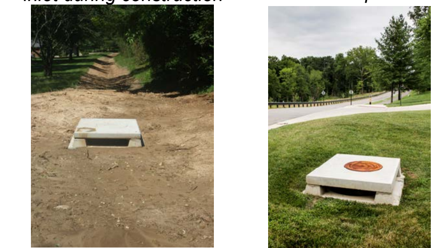
An example single area inlet during construction An example single area inlet completed
