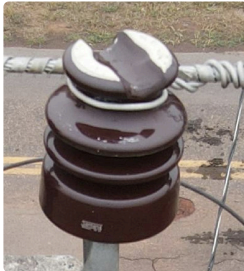
An undamaged ceramic pin insulator used for training an AI-model
