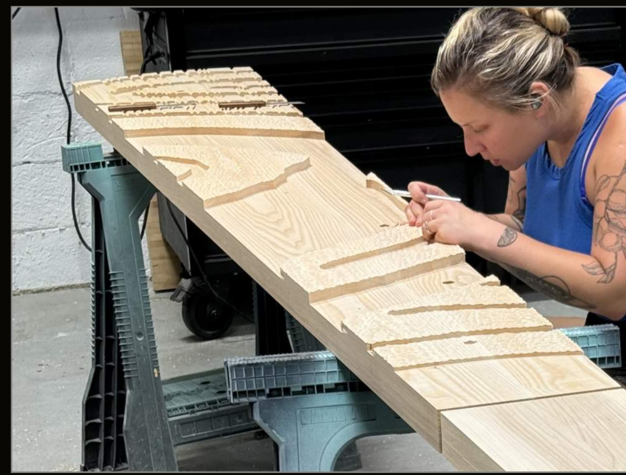
Center The full-scale visual mock-up panel receive patterning before raised wood elements are placed by hand into the recessed grooves shown here.
