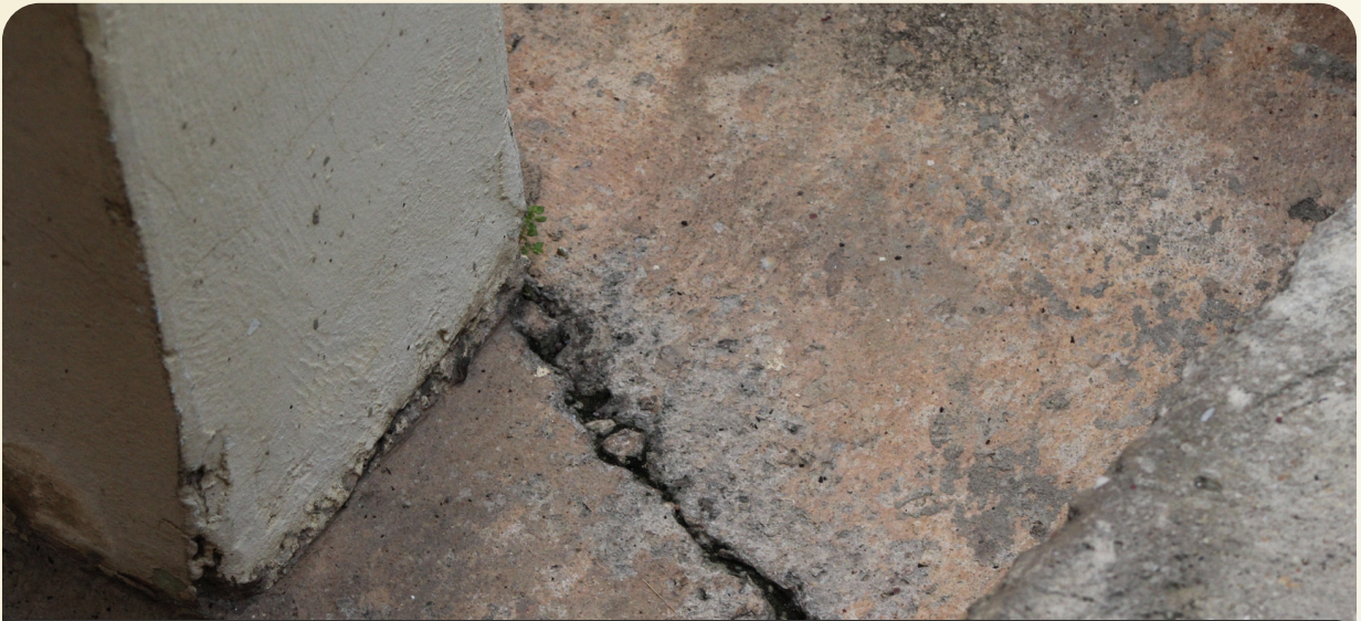
Foundation & Structural Movement
