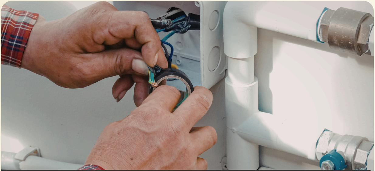
Electrical & Plumbing Problems
