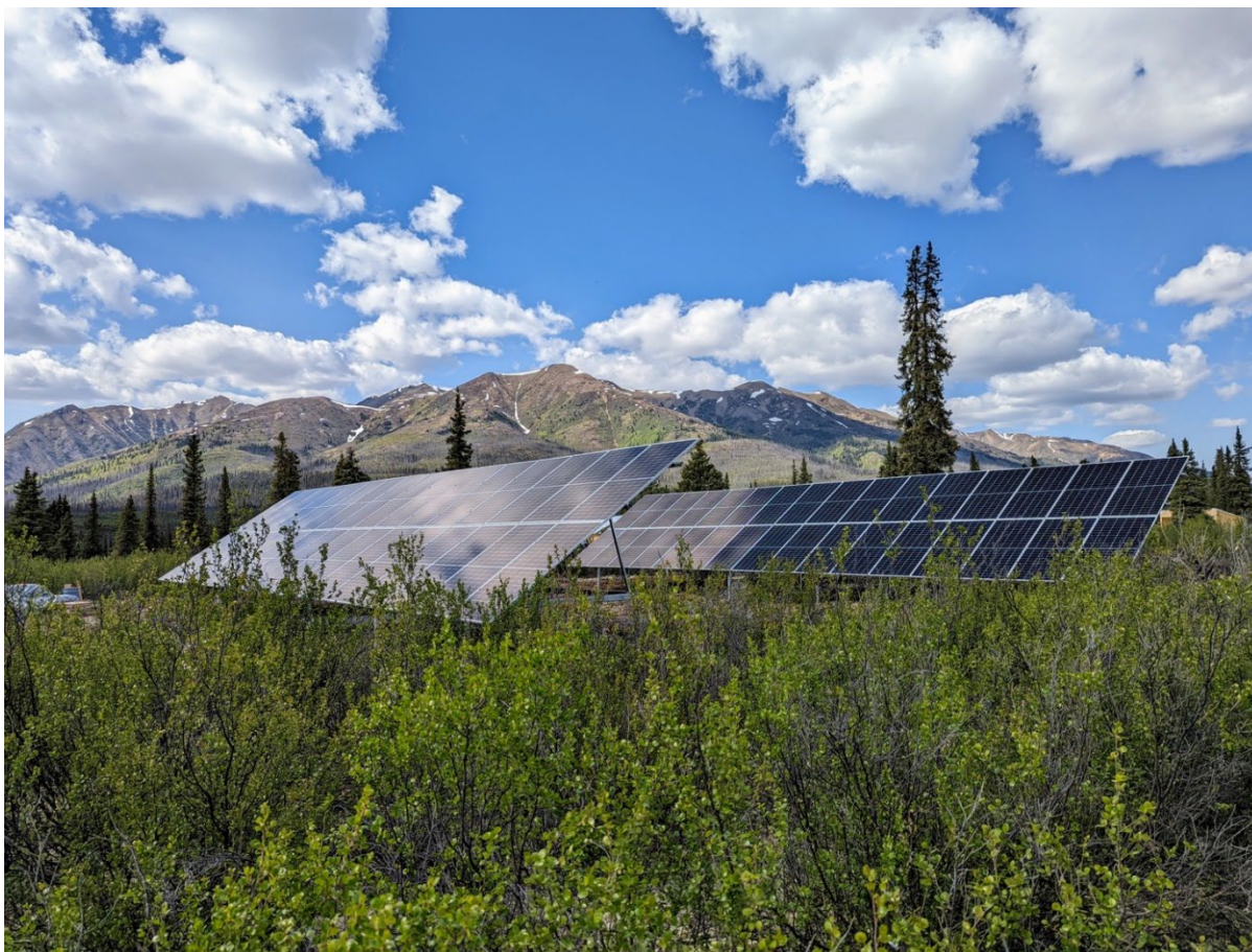
Solar panels in position at Snowline's Forks Camp. Designed by Solvest Inc. the 27-kW hybrid-solar generator system is among the first of its kind to be used to power a remote exploration camp in Canada.
