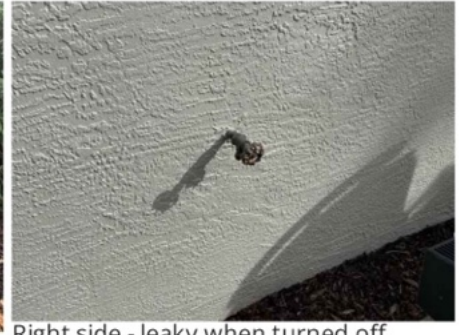
Right side - leaky when turned off
