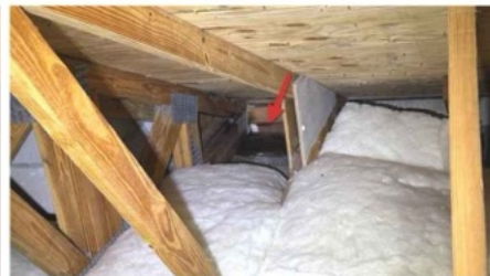
Leak #2 observed in attic in soffit area by chimney above master closet
