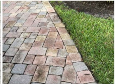
Settlement of edge pavers
