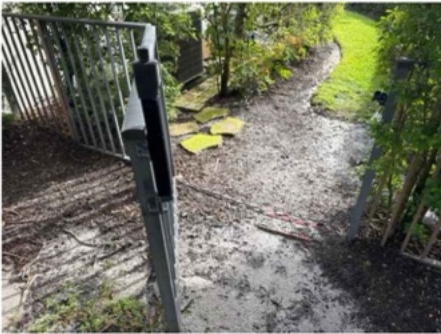
Pool gate not self closing
