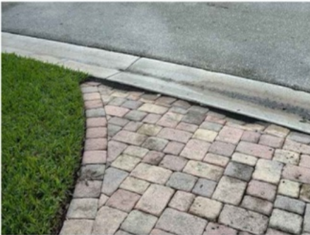
Settlement at street
