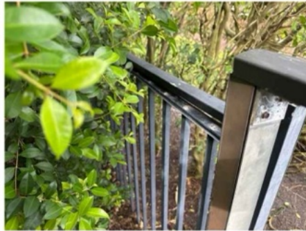
Top rail damage
