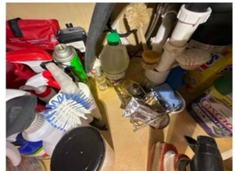
Significant caved in damage to kitchen sink cabinet
