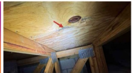
Leak in front of chimney onto living room roof ceiling in front of fire place
