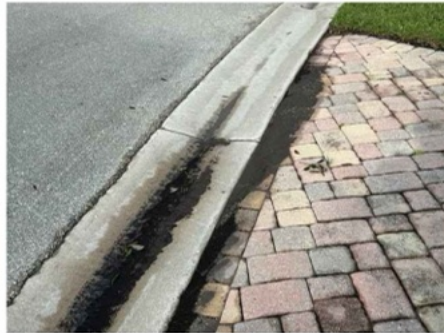
Settlement at street
