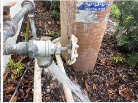
Missing backflow preventer
