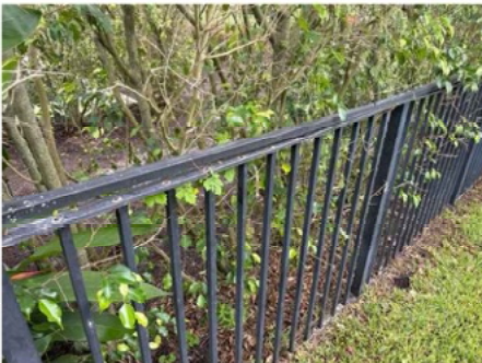
Detached Top Rail Left Side
