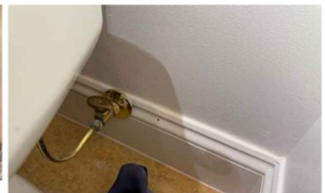
Bidet cold supply shut off at time of inspection
