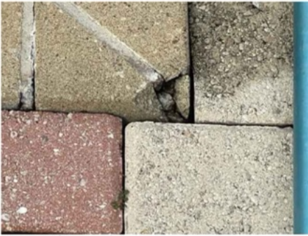
Paver chipped corner
