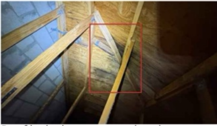
Roof leak above master hatch
