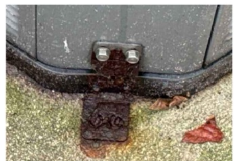
Rusted out hurricane straps
