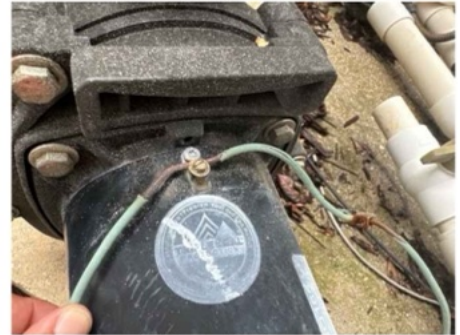
Loose Bond Wore at Pump
