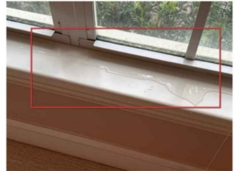
Water on window sill
