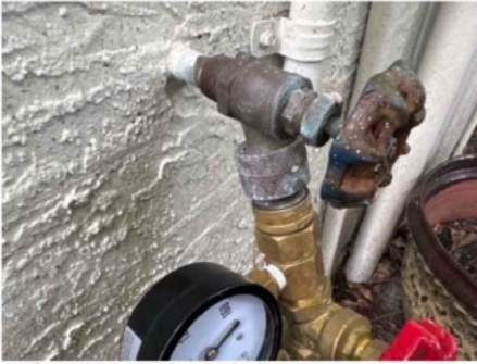
Left Side - Leaky valve stem
