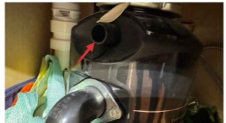
Missing Cap - Island Disposal
