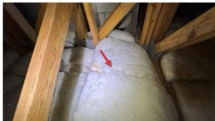
Wet insulation above living room ceiling
