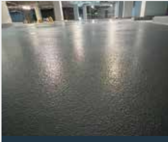
POLYURETHANE COATING FLOORING
