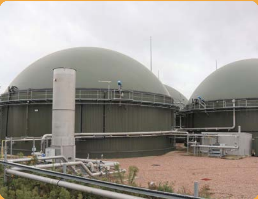
FIGURE 3: A TYPICAL WET-AD FACILITY SHOWING ROUND TANK CONSTRUCTION OF THE DIGESTERS INTO WHICH LIQUID OR LIQUIDIZED FEEDSTOCK IS FED FOR DIGESTION WITHIN THE TANK, EQUIPPED WITH GENERAL MIXING OF THE SUBSTRATE
