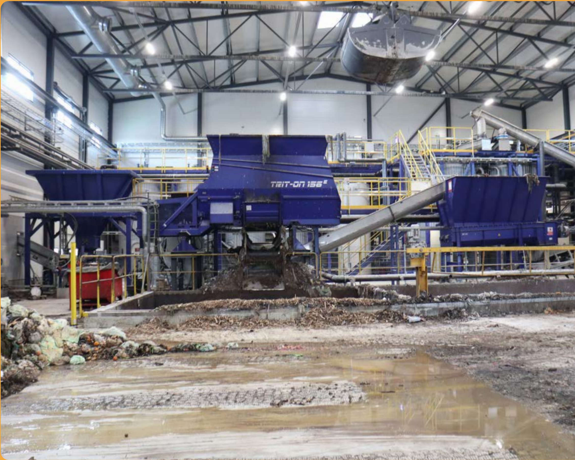
FIGURE 6: DEPACKAGING EQUIPMENT REMOVES ALL PACKAGING FROM FEEDSTOCK
