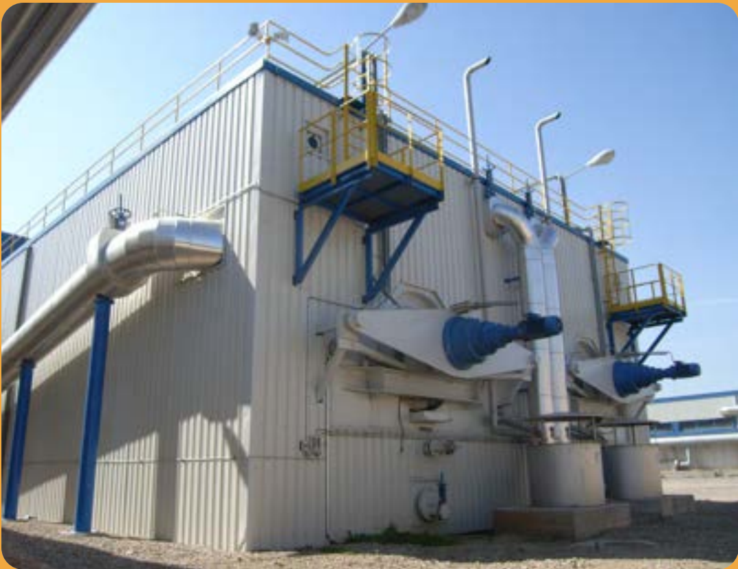
FIGURE 4: A TYPICAL PLUGFLOW HIGH SOLIDS AD (HSAD) FACILITY SHOWING THE BESPOKE NATURE OF CONSTRUCTION INTO WHICH FEEDSTOCK IS FED EITHER AS LIQUIDS OR SIZE-REDUCED SOLIDS TO TRANSIT THE DIGESTER FROM ONE END TO THE OTHER IN A CONTROLLED FLOW THROUGH THE SYSTEM
