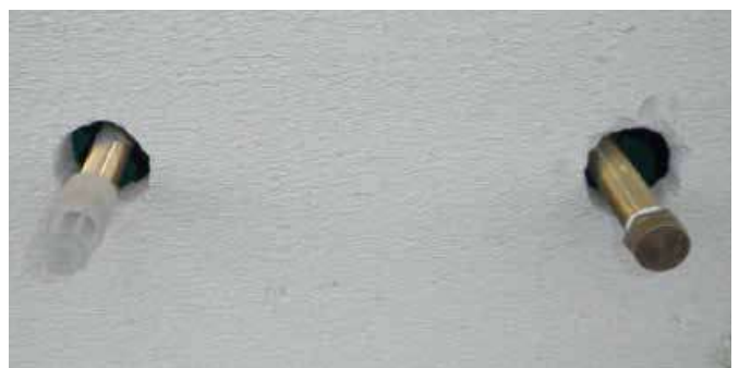
Figure 14.4 Neat finishing of installed services
