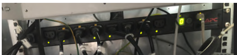
Figure 22: Power bar in electronic cabinet
