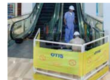
ELEVATOR / ESCALATOR / TRAV-O-LATOR MAINTENANCE
