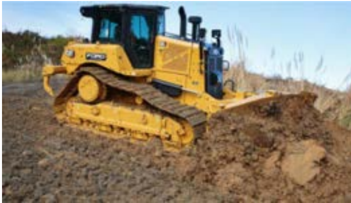
Figure 4: Example of types of bulldozers that would be used for site clearing works
