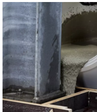
Machine Foundation & Baseplates
