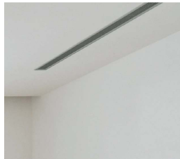
Ventilation grille in the suspended ceiling
