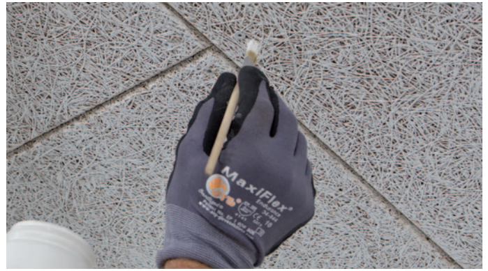
Painting over the screw heads - Use a fine brush to cover unpainted screw heads with the colour of the panels after installation. It is absolutely necessary to avoid double painting of the panel surface around the screw head. This would cause irritating colour differences.
