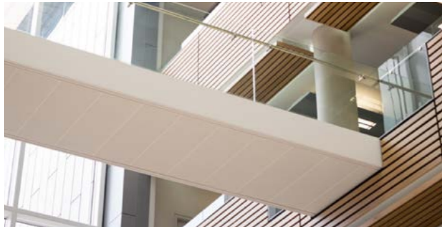
MBS SAS205 System: Corridor Ceiling
