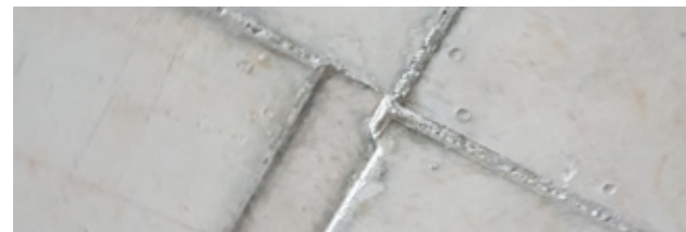
Misaligned formwork was identified as a contributing factor to tension in internal framing.
