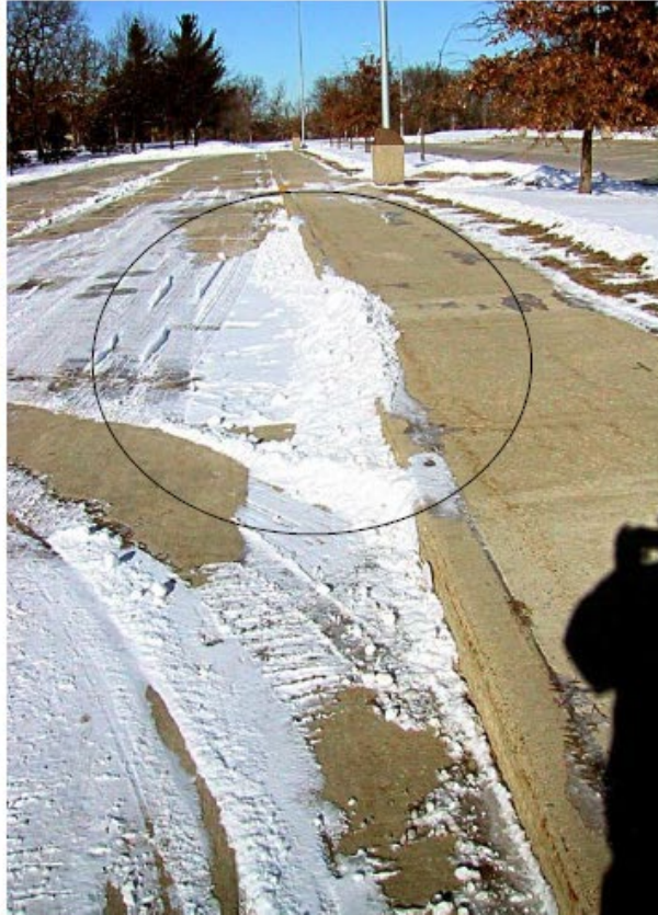
Does Not Meet Standards
