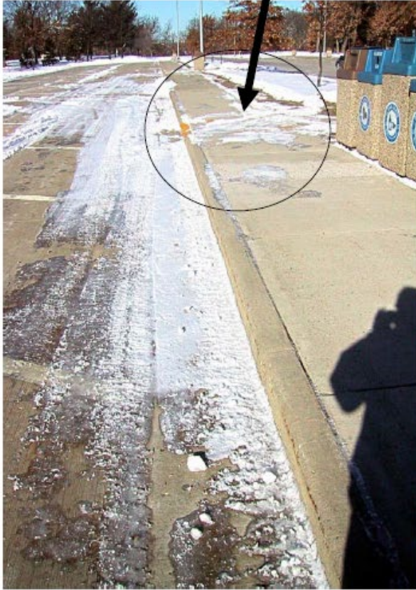
Does Not Meet Standards
