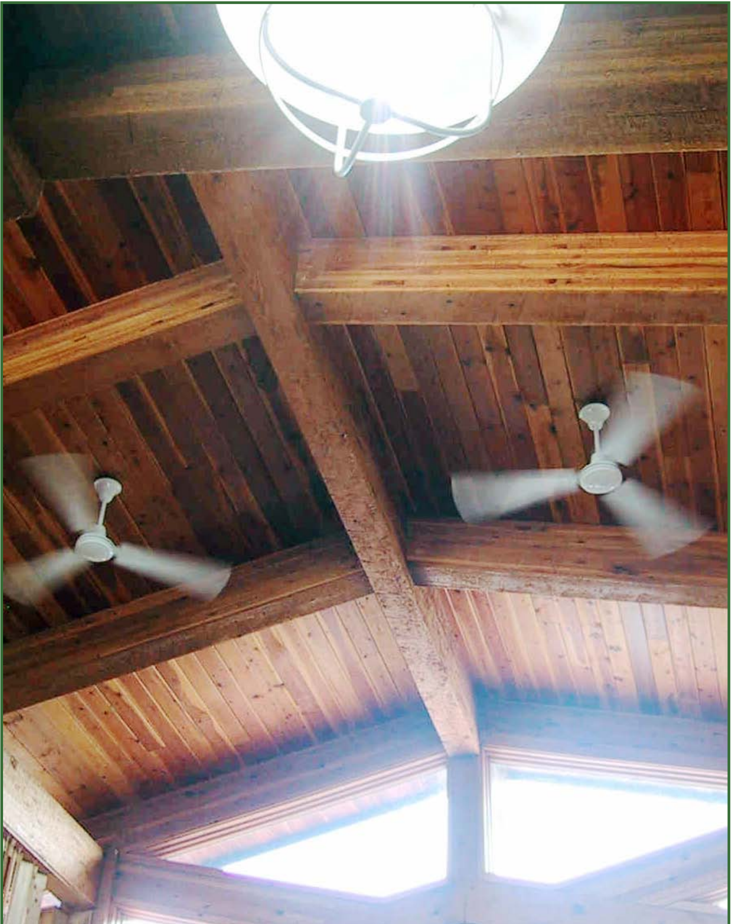
Photo: Iron County TIC 103 in Hurley - New Ceiling Fans Installed in FY 2004 increased the heating and cooling efficiency of the building.
