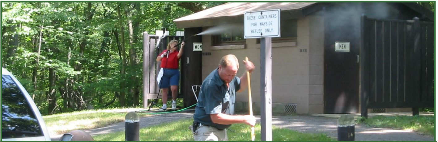
Photo Above: Northwoods Inc., Portage, crew members working at a wayside in Adams County.
