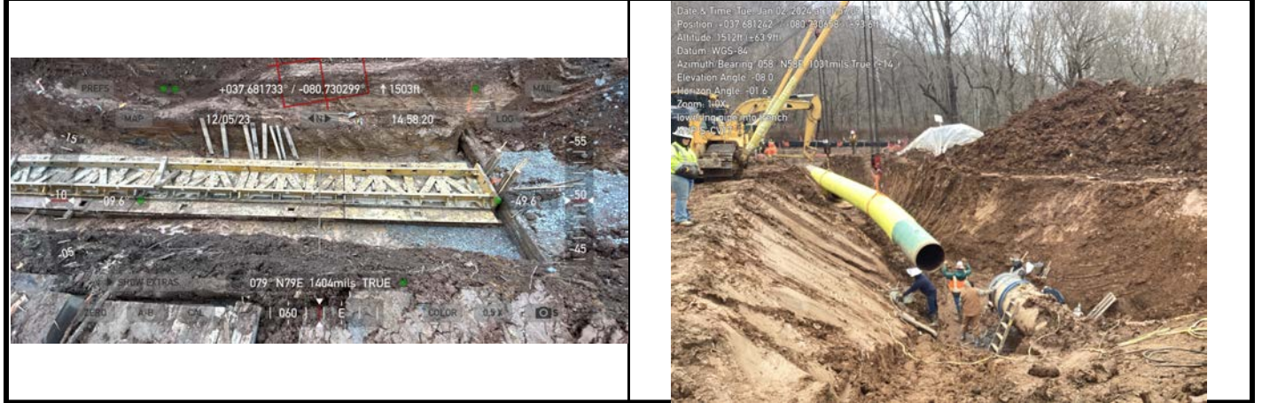
GPS Location See Photo GPS Location See Photo Description Photo 3: Bore tracks in aquatic resource. Description Photo 4: Lowering pipe into trench into aquatic resource area.
