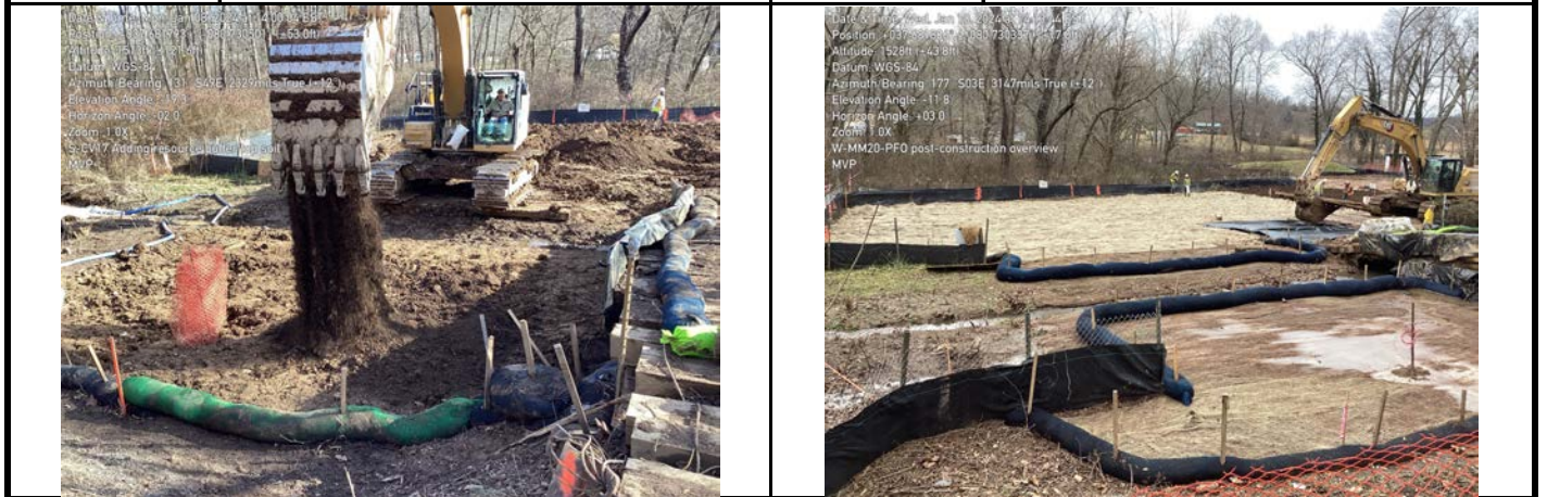
GPS Location See Photo GPS Location See Photo Description Photo 7: Adding topsoil to aquatic resource inside S-CV17 buffer. Description Photo 8: Overview of wetland. Seeding ongoing.
