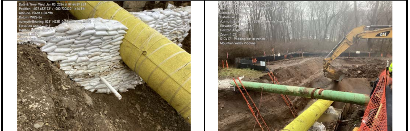
GPS Location See Photo GPS Location See Photo Description Photo 5: Trench breaker constructed with French drain. Description Photo 6: Adding padding dirt and backfilling trench.
