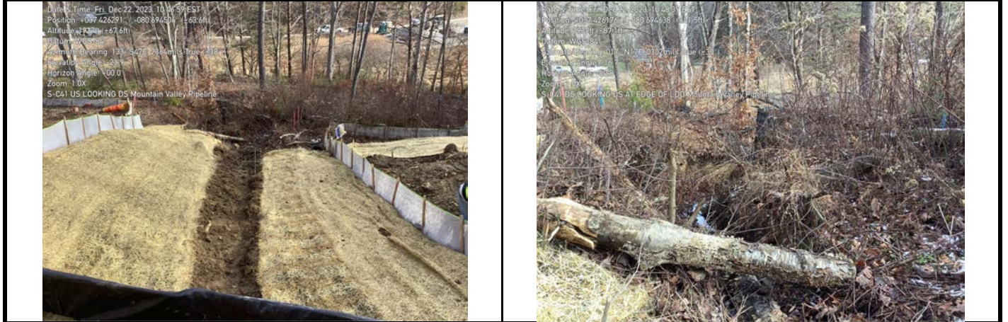
GPS Location See Photo GPS Location See Photo Description Downstream view of permitted impact area during post-construction assessment. Description Downstream view of unimpacted area during post-construction assessment.
