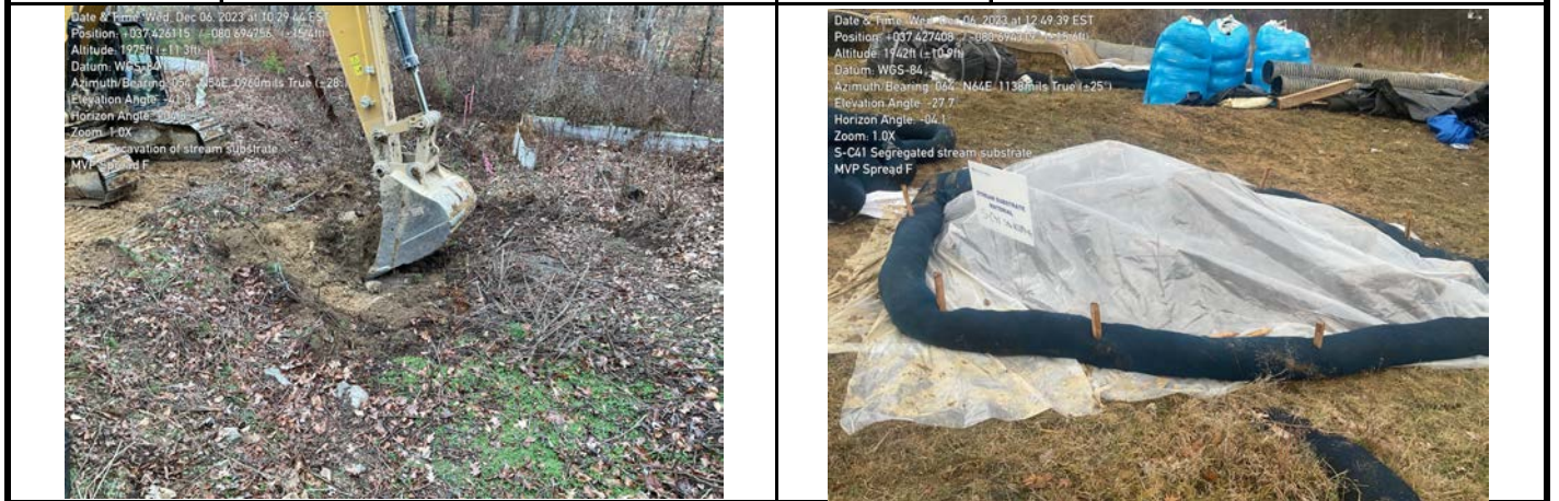
GPS Location See Photo GPS Location See Photo Description Photo 1: Excavating top 12 inches of substrate. Description Photo 2: Substrate segregated and stored in upland area.
