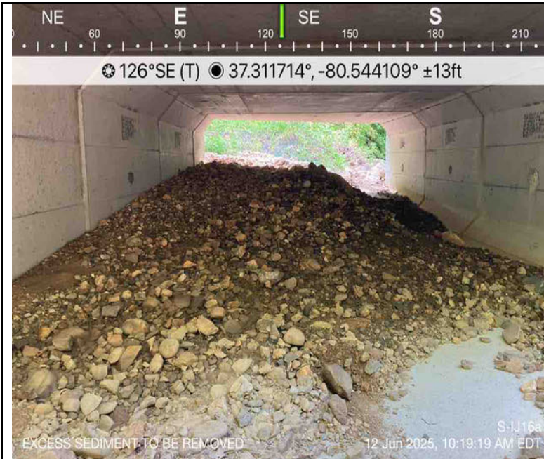
Photo Description: Culvert full of excess substrate inhibiting flow.
