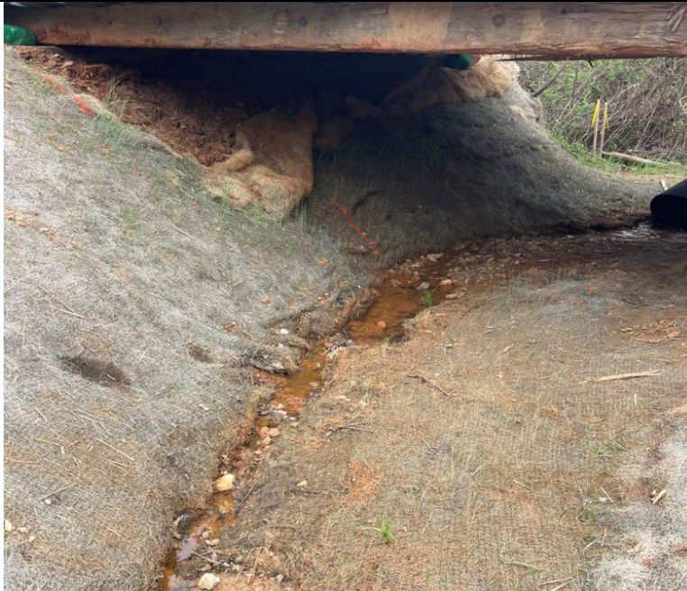
Photo Description: Downstream view of permitted impact area during pre-construction assessment. No GPS data available.
