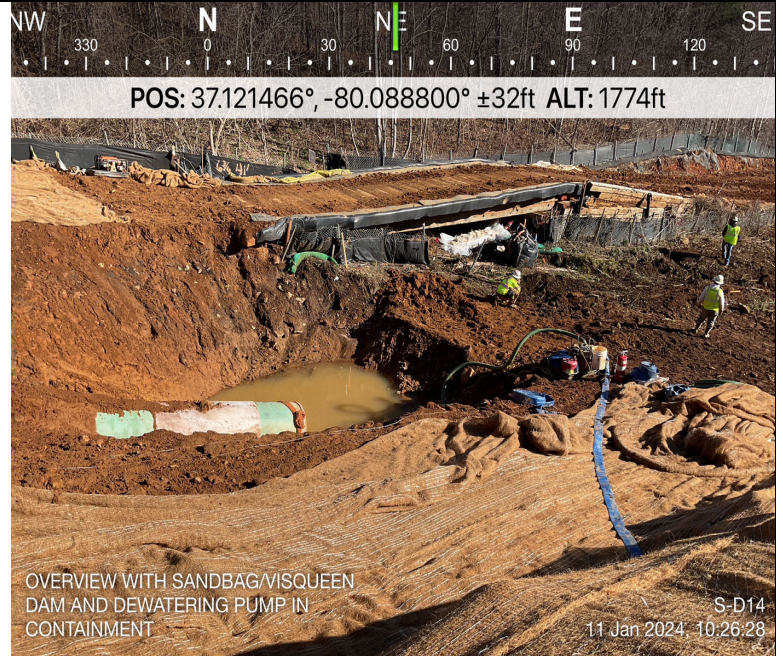
Photo Description: An overview of the sandbag and Visqueen dam.
