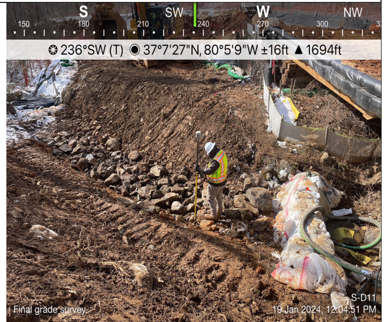
Photo Description: Survey shooting final grade after restoration of the stream substrate.
