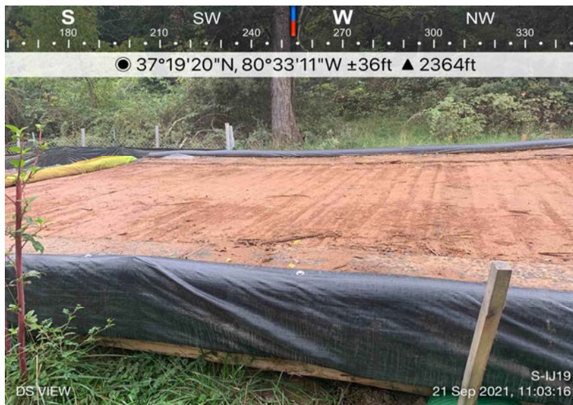
Downstream view looking S within access road. Stream was not found in the field, however, riparian buffer scores were assigned based on best professional judgement. Assessment is limited to areas within the temporary ROW.
