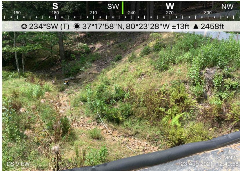
View downstream looking SW. Assessment is limited to areas within the temporary ROW.
