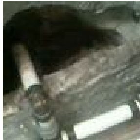
10-2e Hole in wall to water line
