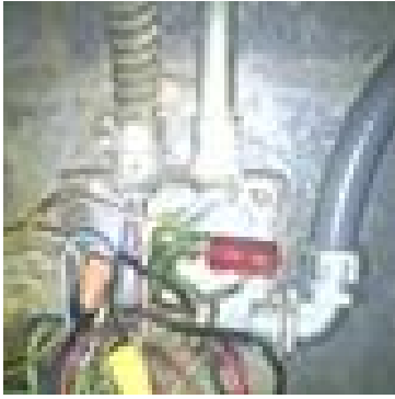
10-5g Contractors leave wires exposed
