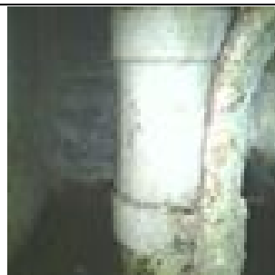
5-2k Rust all over beds
