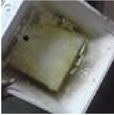
10-4e Mildew on mop closet tub
