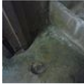
10-4f Mop closet mold enters living area
