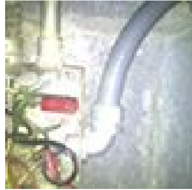
10-5h Shabby contractor work
