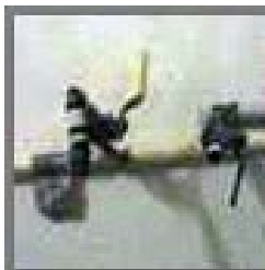
4h Broken shower head
