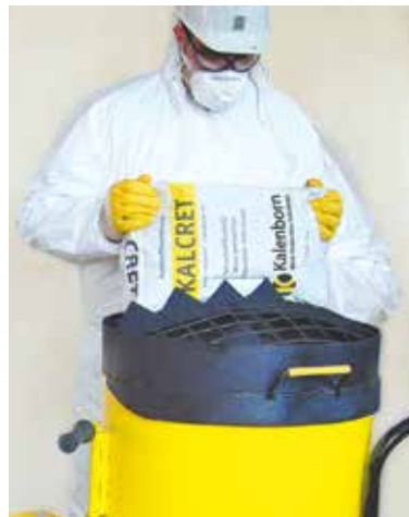
Material feeding into the forced circulation mixer
