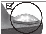
OVAL NECK OF BOLT SEATED PROPERLY
