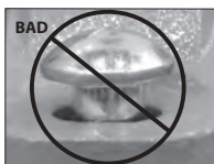
OVAL NECK OF BOLT NOT SEATED PROPERLY
