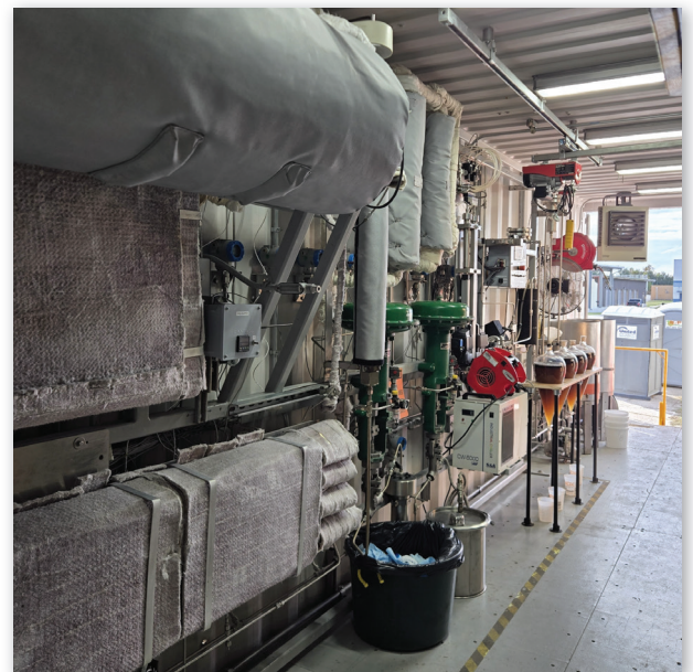
Genifuel HTL pilot system equipment.
