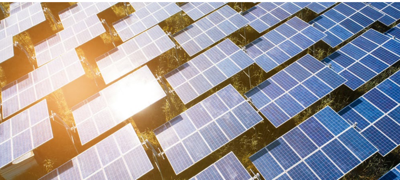
📍 Solar panels, Queensland
